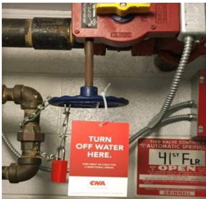
CNA Water Valve Tag Photo Source: CNA Insurance
